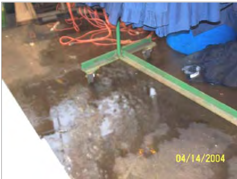
Another aspect of the wet floor at the Municipal Garage as a result of the rain coming through the roof.
