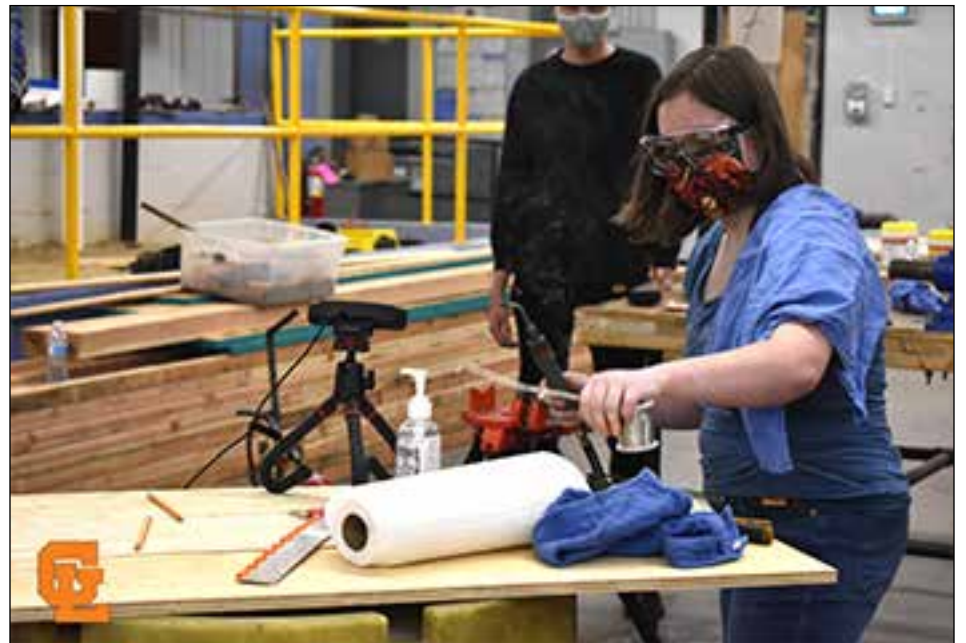
Kaitlyn Distefano, a GLTS freshman from Methuen, learns how to solder pipes on her first day of in-person learning in plumbing. She is one of over 200 freshman students who began learning in-person for their exploratory courses this week. (Photo courtesy of Greater Lawrence Tech)
