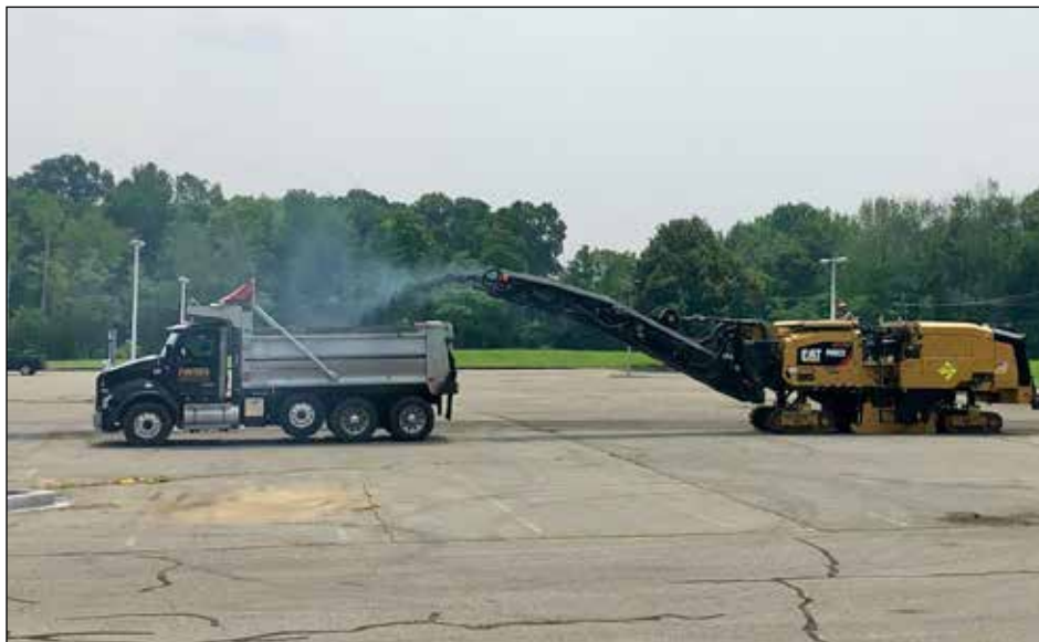
With $1.5M in funding from the Massachusetts Department of Capital Asset Management and Maintenance (DCAMM), parking lots that have suffered from frost heaves, pot holes, and crumbling asphalt are being completely resurfaced.
