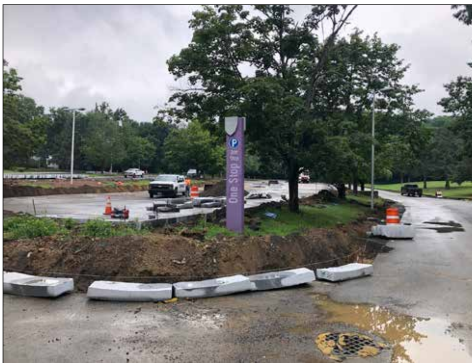
After decades of being battered by weather, traffic, and snow plows, all of the curbing around campus is being replaced with brand new New Hampshire granite!
